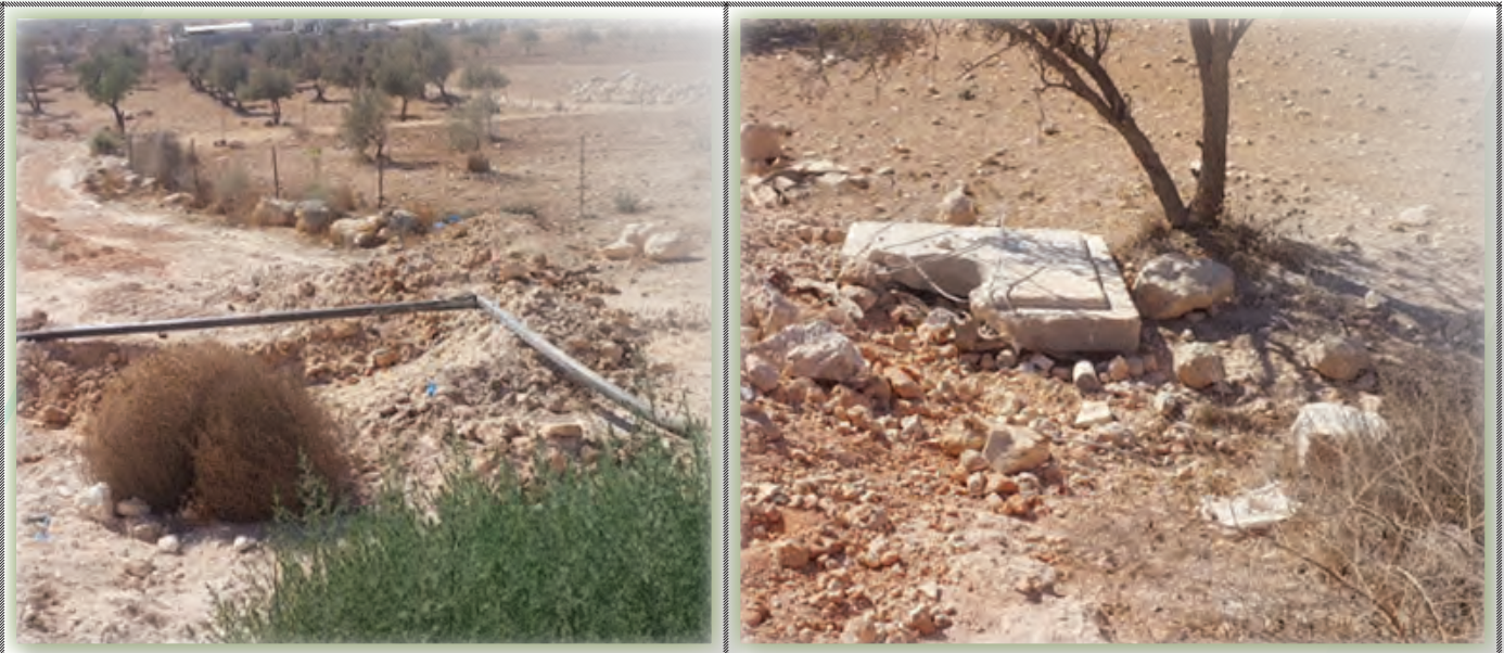
Damaged water network Infrastructure following Israeli demolition in Zif – 2025
